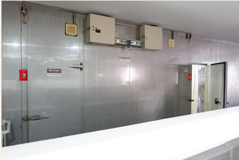
Walk-in Freezer and Chiller
